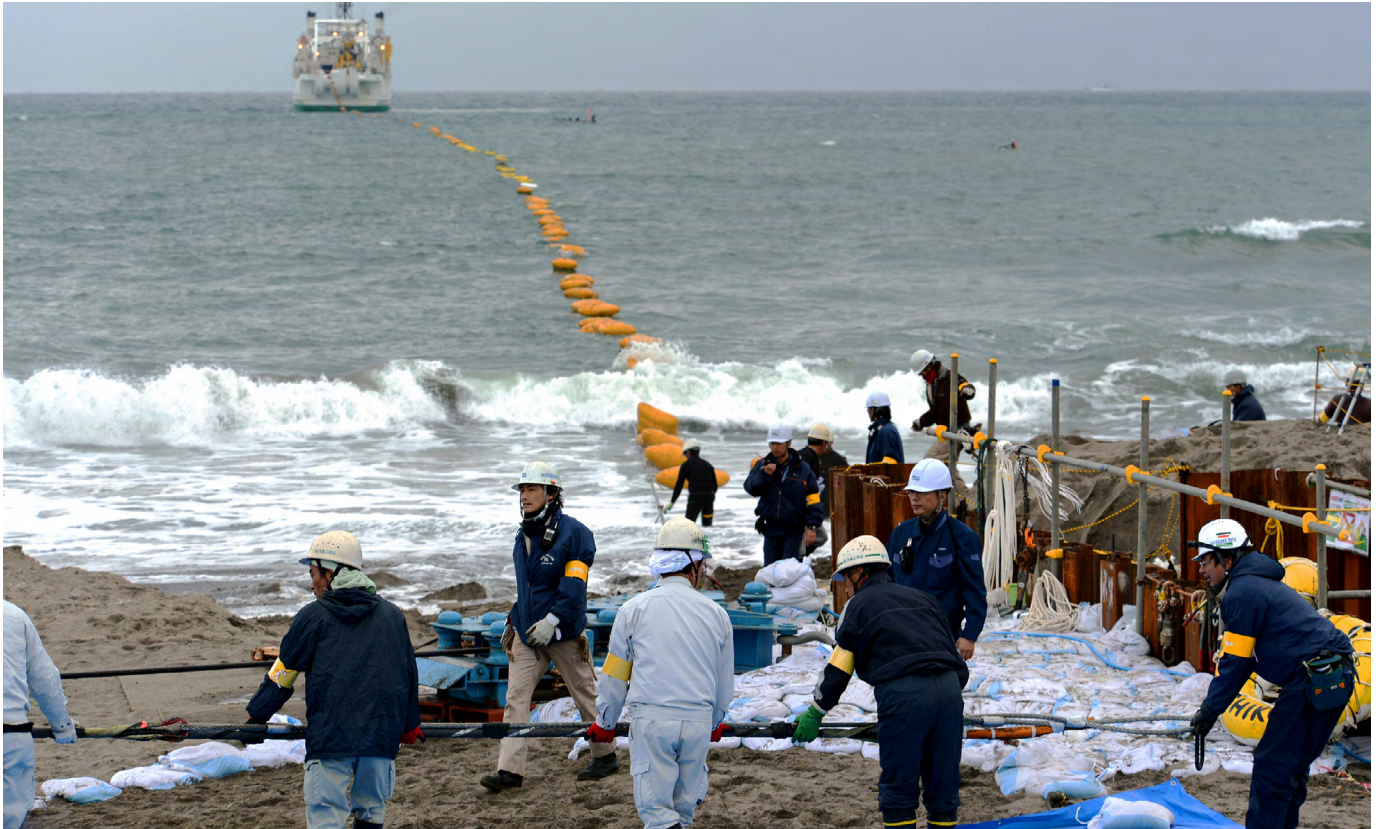
Workers pull an undersea fiber-optic cable from a ship, as KDDI Corp. began an operation to lay a cable connecting Japan and Singapore. Photo by The Asahi Shimbun via Getty Images
